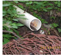
Aeration discharge pipe into a receiving stream
