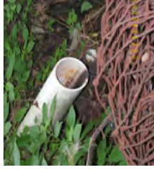
Aeration discharge pipe into a receiving stream
