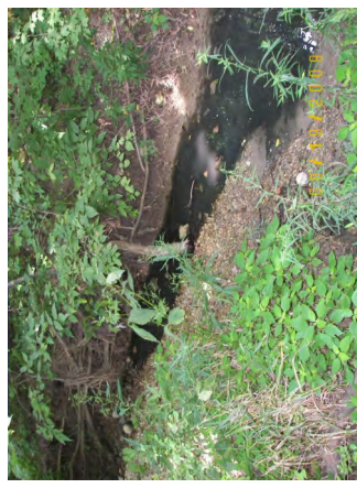
Polluted receiving stream from septic discharge
